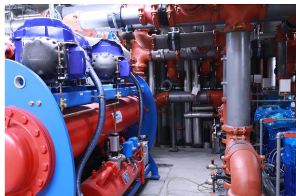
Renewal refrigeration UZA II
